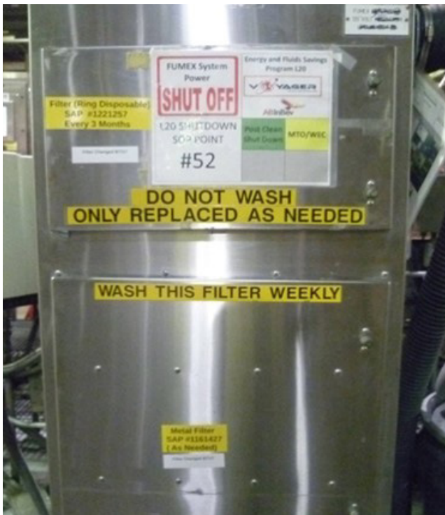
Figure 1. Filter housing of the LEV unit. The top compartment holds the disposable filter and the bottom compartment holds the washable filter. Photo by NIOSH.
