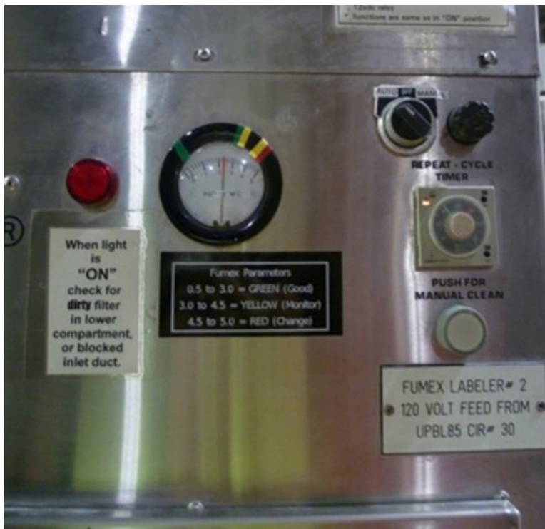
Figure 2. The controls and filter pressure drop gauge on the front of a LEV filter housing unit. The gauge is labeled with ranges where the filter performance is “good” (green), should be “monitored” (yellow), or should be “changed” (red). A knob on the top right shows the current LEV mode as “auto” or “manual.” Photo by NIOSH.
