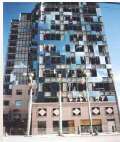
2005 Hurricane Wilma damages Broward County School Board Building Source: Photo by Susan Gillis, Historian
